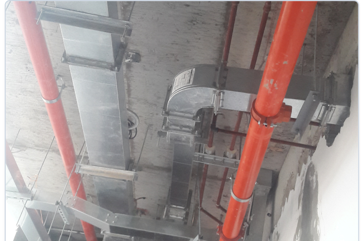
Overhead fire sprinkler distribution piping and central HVAC ductwork
